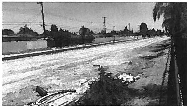
Here's current (mid-May) view of the trail under construction, along the east side of Brookhurst. Grading is complete, so paving for the bike trail and installation of decomposed granite for the walking path are next.
